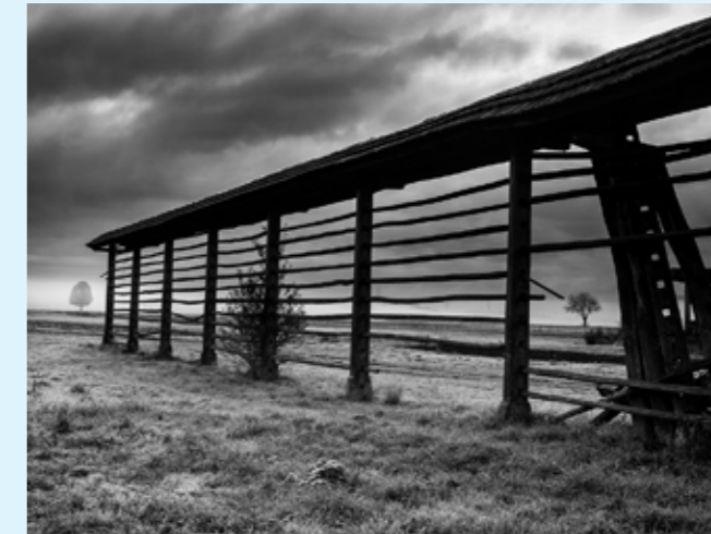
This hayrack is in bad condition, some bars are already broken
